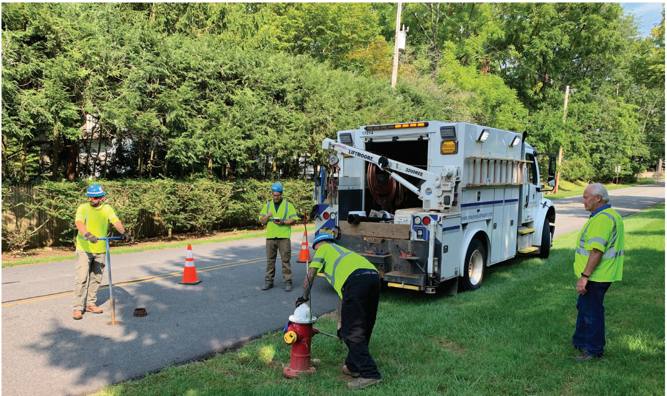
FIGURE 4: NJAW PERFORMING THE INSTALLATION OF THE SENTRYX SOFTWARE ENABLED SUPER CENTURION HYDRANT PRESSURE MONITORING RETROFIT KIT.
